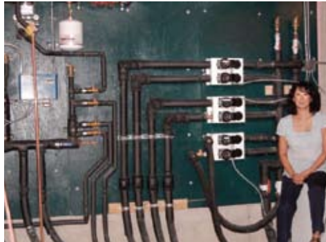
Karen Casey stands besides her basement "green" wall, which cuts the electric bill from $750 a month to $21.
