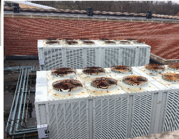
A successful referendum would protect the community's investment in school buildings by repairing and renovating aging building conditions at all schools. Pictured: HVAC units at BMS-Prairie.
